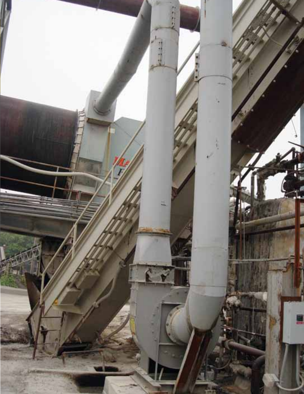
Here a high CFM fan pulls errant smoke off the slat conveyor for return to the burner and incineration. Photo courtesy of Murphy Pavement Technology, Chicago.
